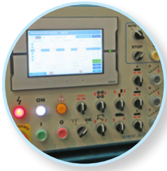
CMC Control Panel
