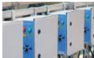
Panel de control central
